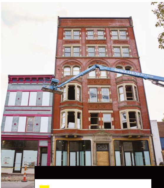
GOING UP Construction is underway on Phase 1 of the Trevarren Flats project (two of the three buildings are shown here).
